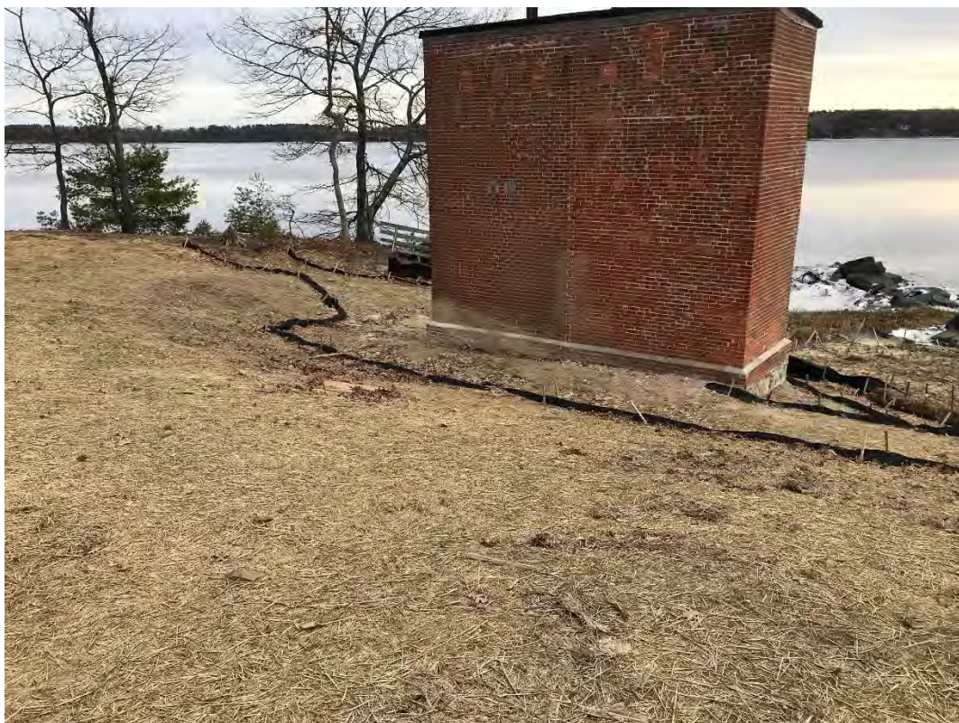
Fig 2: Slope leading down to cable house and salt marsh restoration at the Eversource property/west side of the bay. Viewing northeast. (12-30-20)
