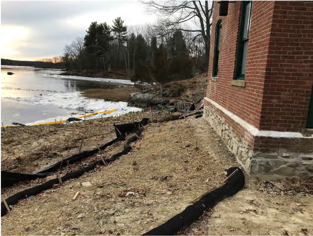
Fig 3: Slope between the cable house and salt marsh restoration at the Eversource property/west side of the bay. Viewing south. (12-30-20)
