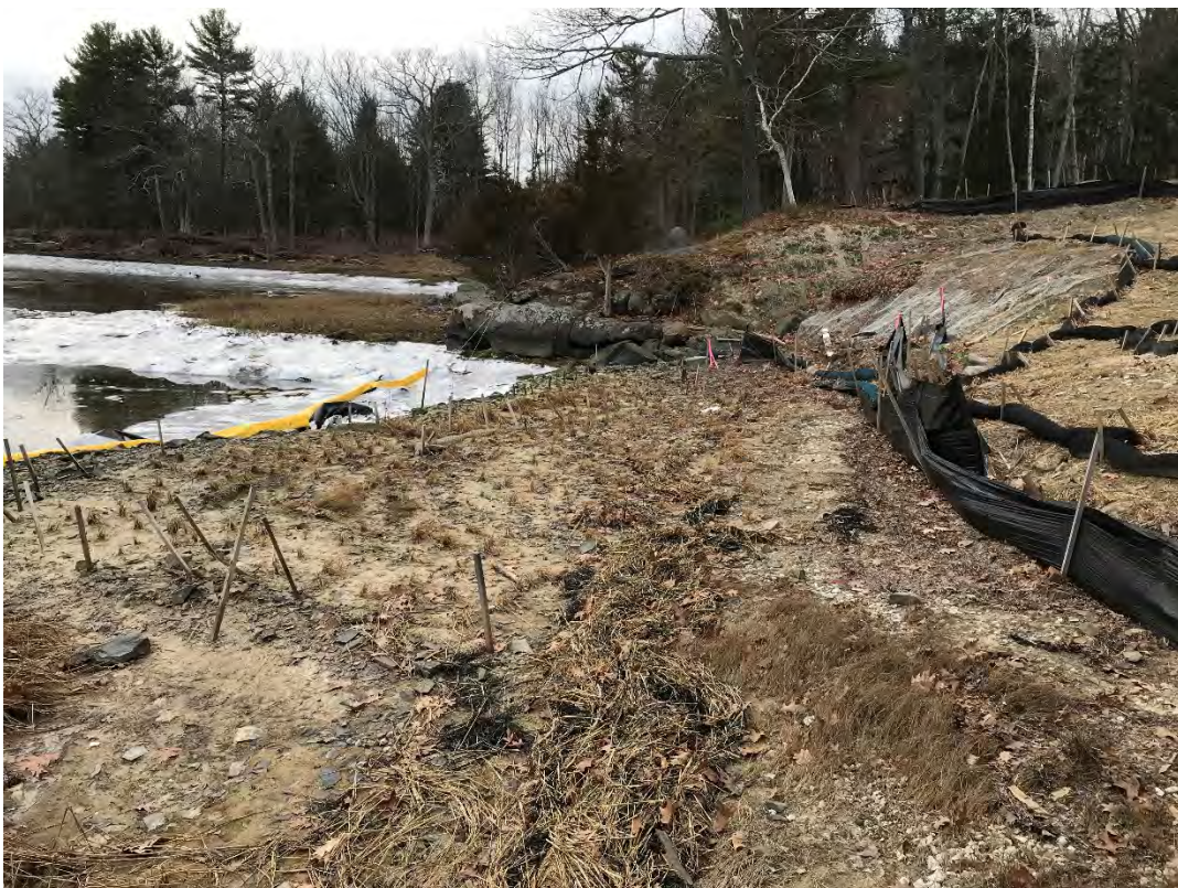
Fig 4: Toe of the slope and salt marsh restoration at the Eversource property/west side of the bay. Viewing south. (12-30-20)
