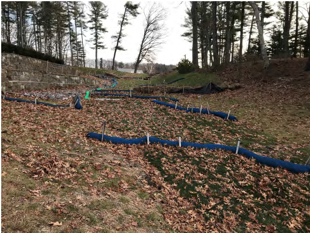
Fig 10: Slope below the manhole at Gundalow Landing/east side of the bay. Viewing east. (12-30-20)
