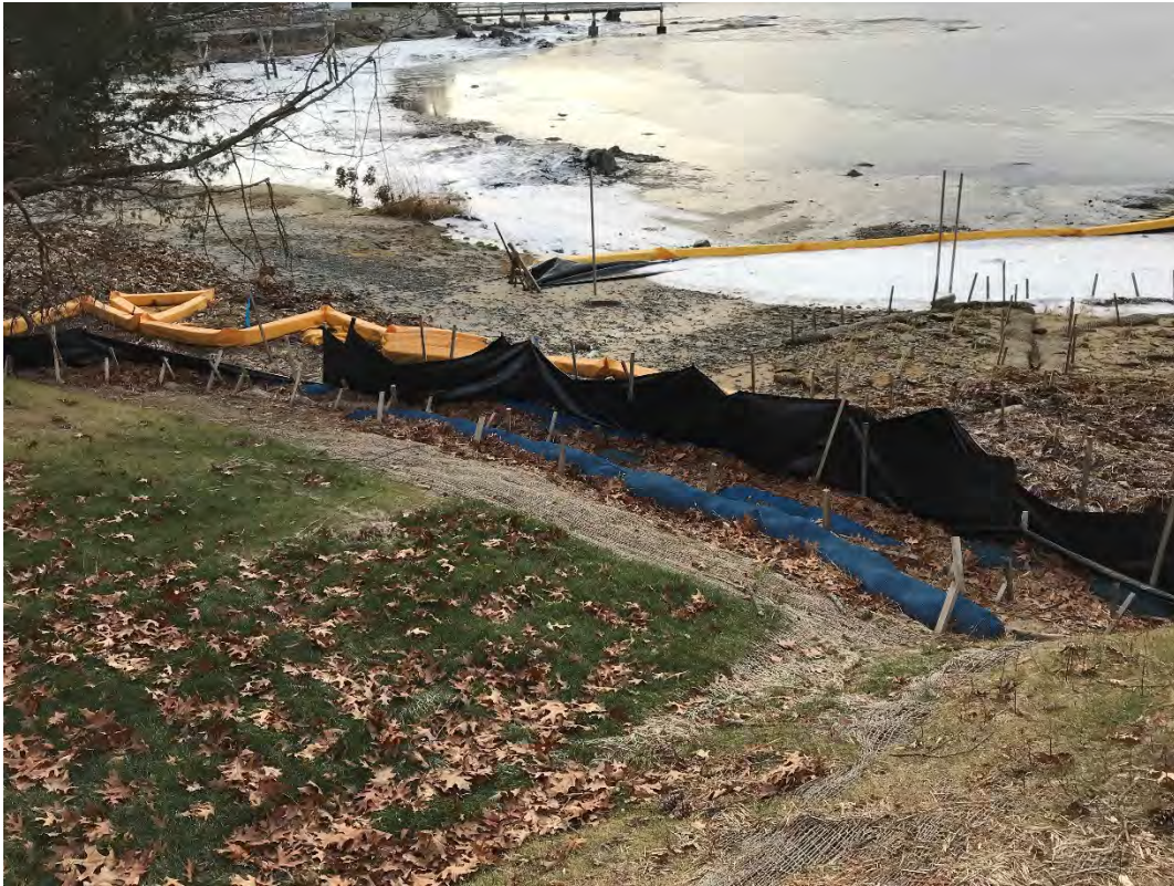
Fig 11: Toe of the slope at Gundalow Landing/east side of the bay. Viewing south. (12-30-20)
