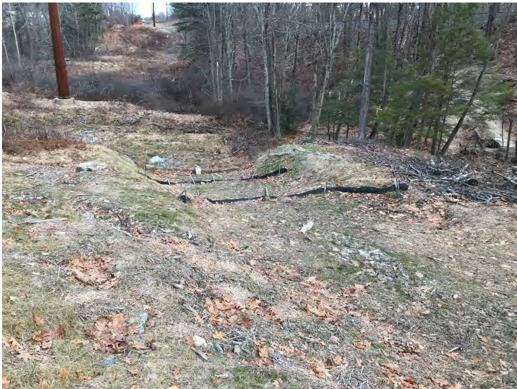
Fig 8: Lower portion of slope between Strs. 28 and 29. Viewing northeast. (12-30-20)
